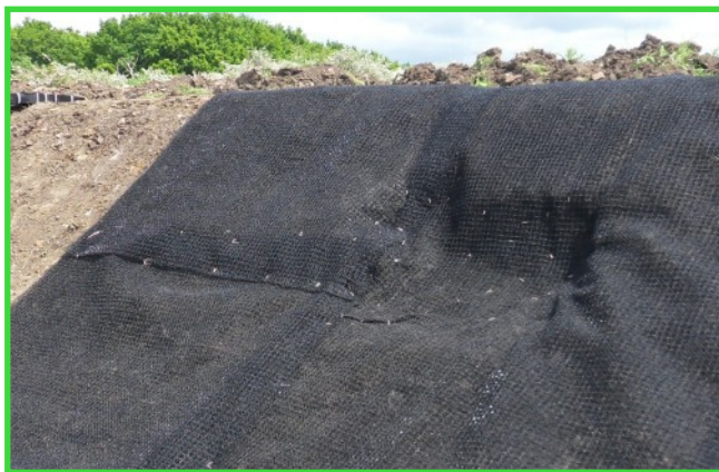
Fig 5: Ensure GeoMat is in intimate contact with the ground IN ALL PLACES
