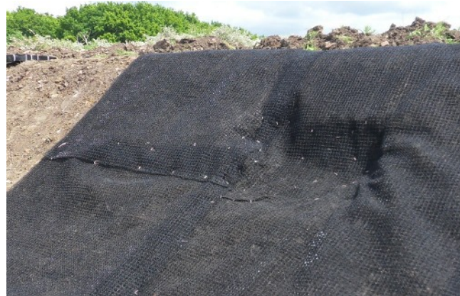
Fig 5: Ensure GeoMat is in intimate contact with the ground IN ALL PLACES
